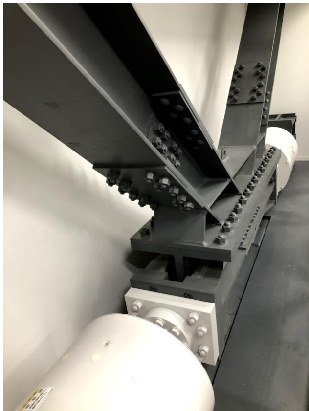
Damping device of NTT East Sendai Aobadori Bldg.
